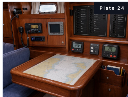
Plate 24. Chart table, VHF/DSC, and electrical panels; tidy and labelled.
