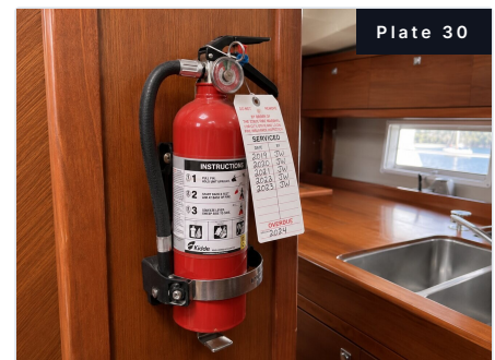
Plate 30. Galley extinguisher; charged, service tag overdue (C-12).
