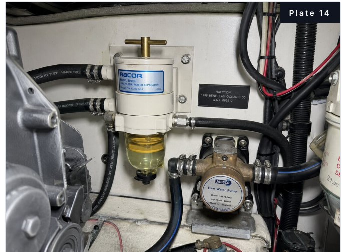
Plate 14. Racor primary separator and raw-water pump; serviceable, double-clamped.
