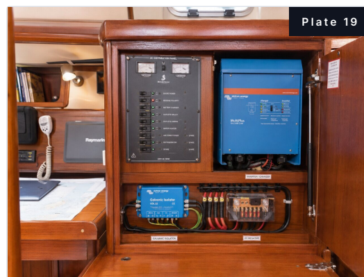
Plate 19. AC distribution, inverter/charger, and galvanic isolator at the nav station.
