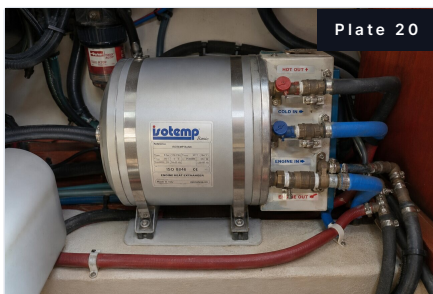
Plate 20. Calorifier and fresh-water manifold; serviceable, no leaks.
