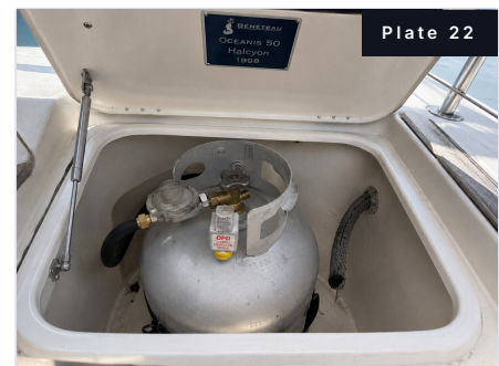
Plate 22. Vented propane locker; overboard drain hose deteriorated (A-2).
