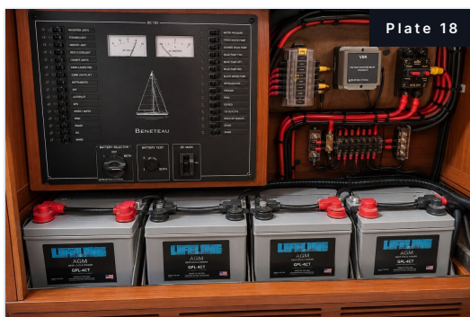
Plate 18. Main DC panel and AGM house bank; tidy, labelled, recently renewed.
