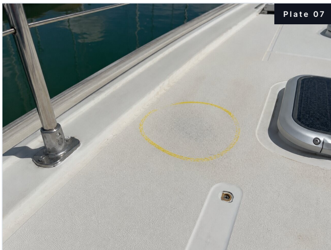
Plate 07. Port side deck; chalk marks indicate area of elevated moisture (Finding B-3, reading 62).
